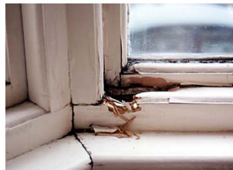
Rotting window frames will be replaced
